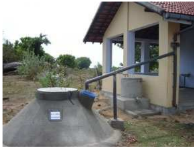
20 m 3 - partial underground tank at Maha Oya school (2)
